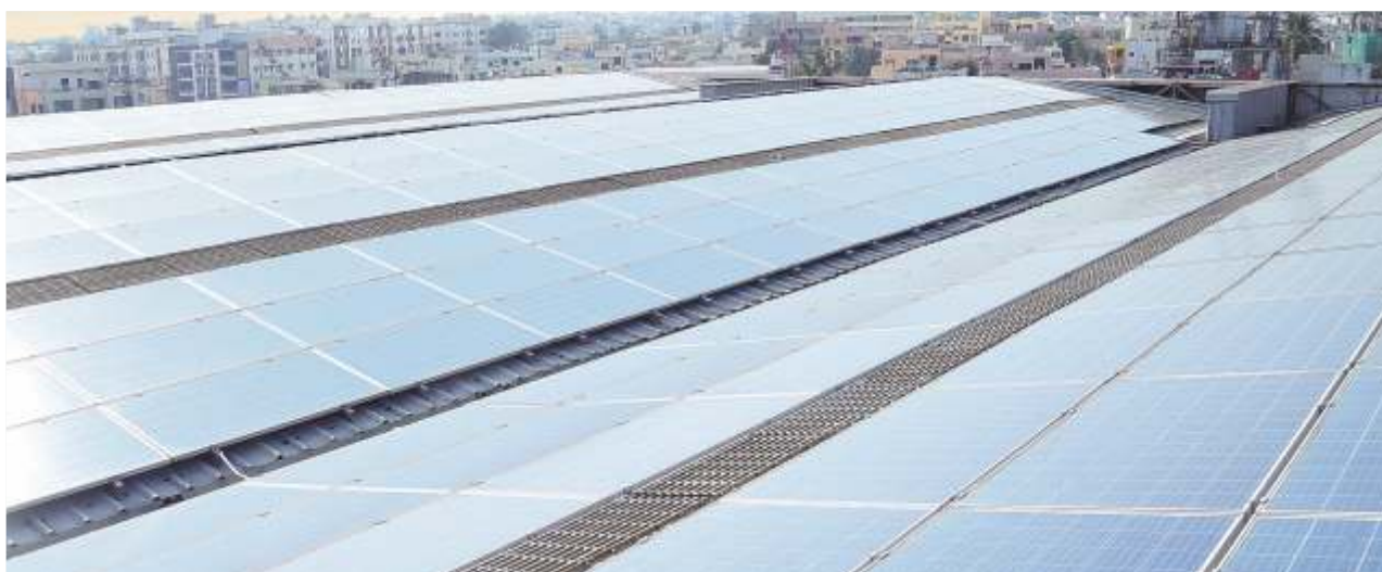
Figure 21: SPAR Hypermarket roof top solar power plant
