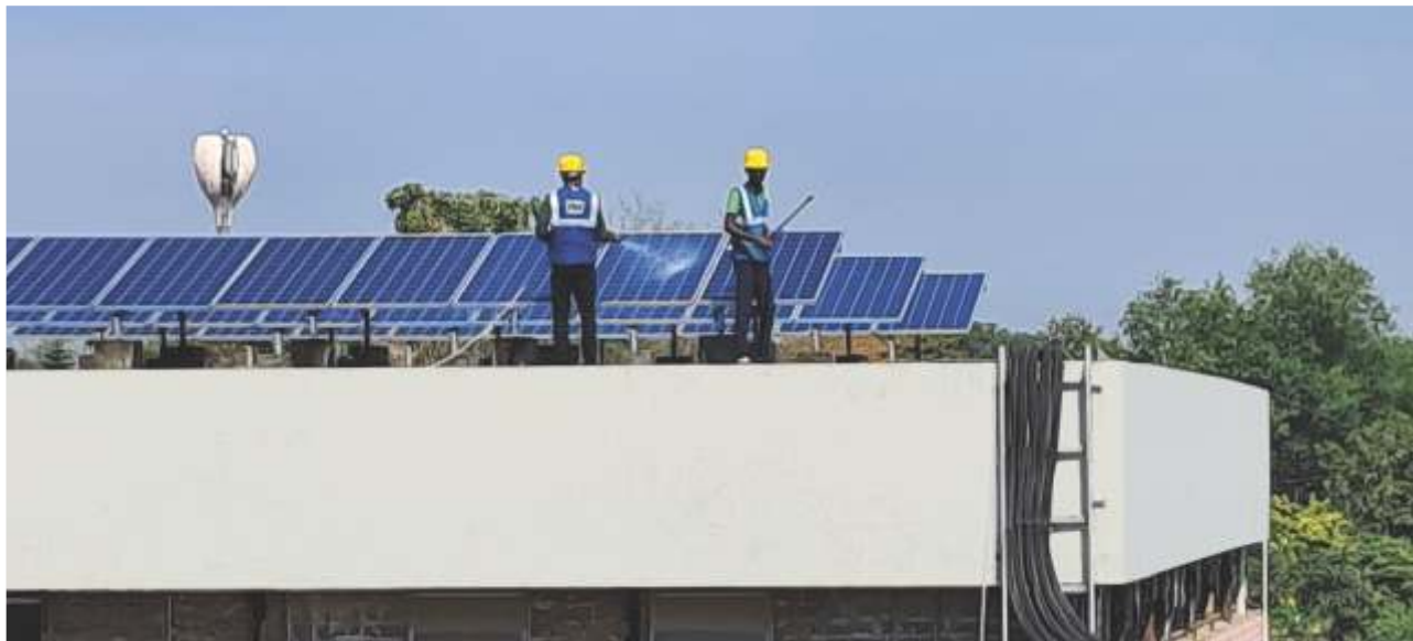
Figure 9: The Tribune solar power plant being cleaned
