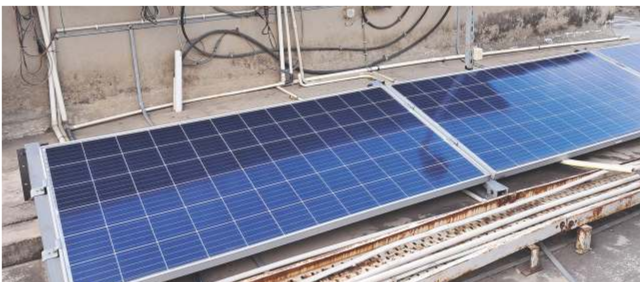
Figure 11: LPS solar grid tie inverters
