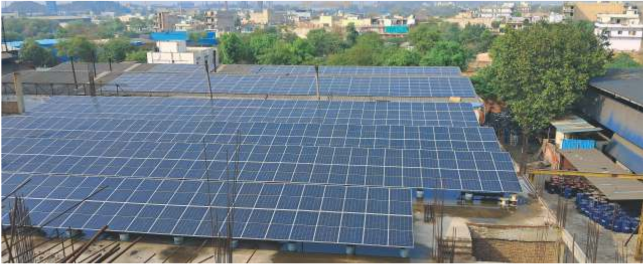
Figure 32: Solar power plant of 430 kWp capacity at Nagdev Industry
