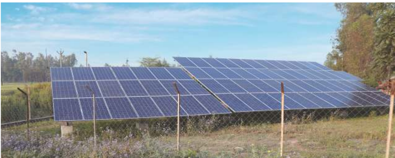
Figure 14: OMC mini-grid power plant at Hardoi (Uttar Pradesh)
