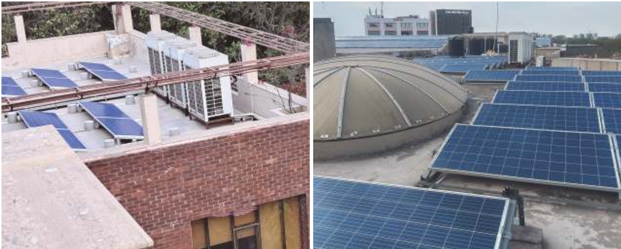
Figure 10: LPS solar power plant of 82 kW
