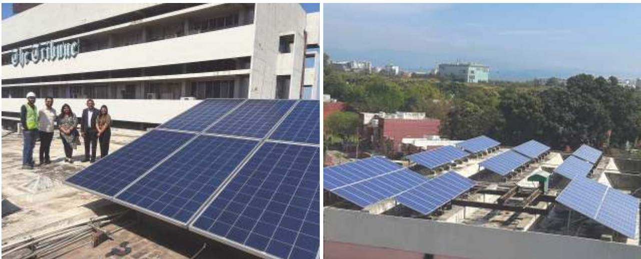
Figure 8: The Tribune solar power plant visited by CPI and OPM, along with Candi Solar representatives
