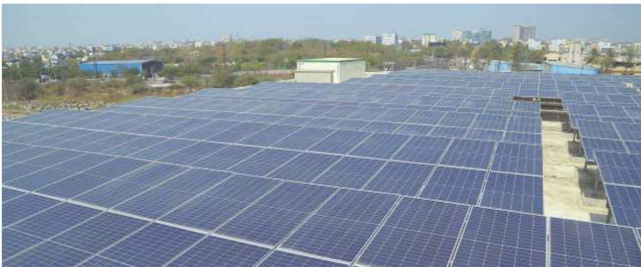
Figure 25: 547 kW plant installed at DMART rooftop by 4PEL
