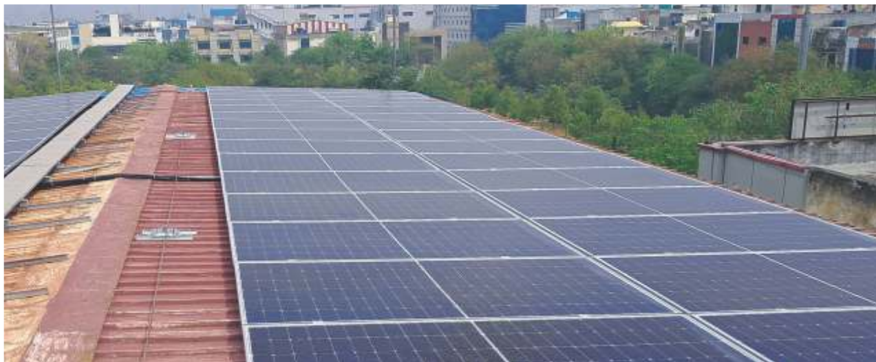
Figure 30: 40 kW on-grid solar power plant of Allianz Exports
