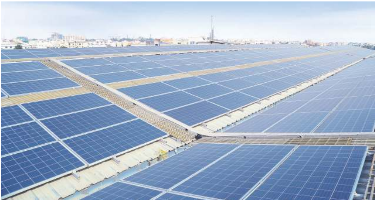
Figure 3: Mini-grid power plant (courtesy, OMC Power)
